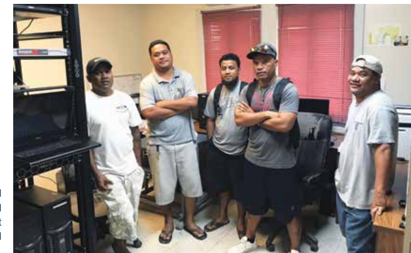
Lincoln Laboratory interns, assisted by Ranny Ranis (far right) completed installation of a server rack as a first step to improve data storage and retrieval at the Ebeye Hospital.
